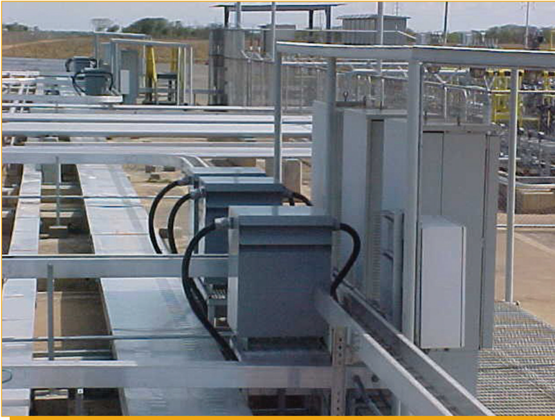
Figure 6. Three Lineators operating with 375 kW (500 hp) pump drives.
