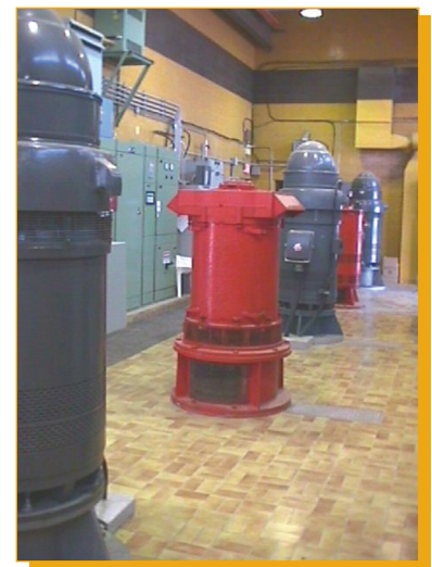
Figure 1. Municipal waterworks – a typical pump application.
