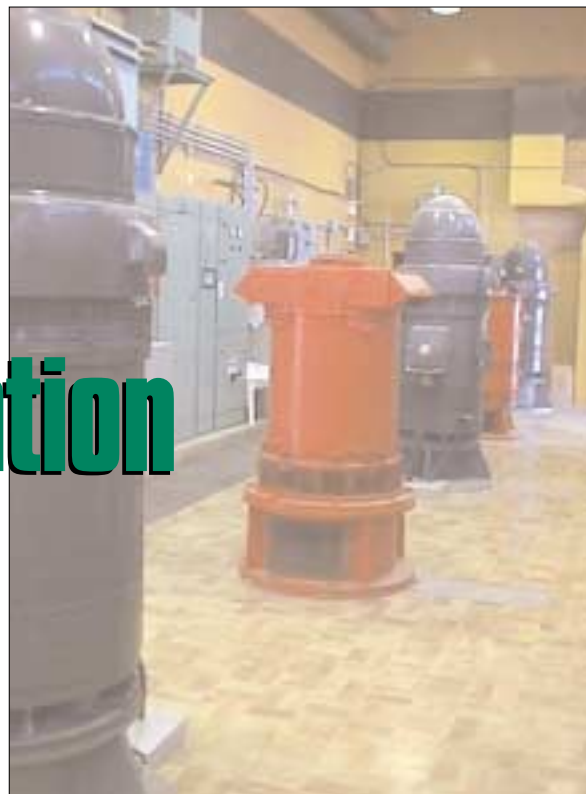
Above: Water pumping station with variable speed pumps
