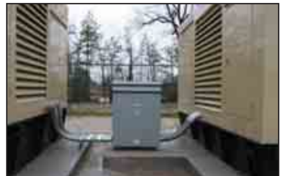
Figure 9: Photo of multiple winding reactor installation.
