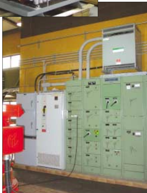
Above: AC variable frequency drives are now commonplace throughout the world, covering the complete spectrum of sectors from air conditioning through to process industries, pumping systems.
